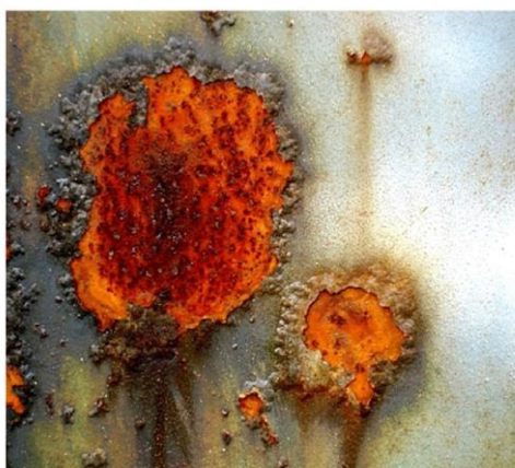
Fig.2. Corrosion on steel surface (Md Shamsuddoha et al, 2013).
